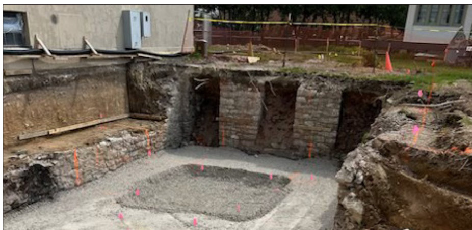
Pictured here are the initial excavations which accommodate the footprint of the new building addition at the history Museum. Existing former stone foundation walls are evident from previous buildings at this site and will stay in place. The new compacted, crushed stone base will provide the pad for the new footings and foundation walls that will allow for the new elevator shaft construction as well as the new egress stairway construction.
